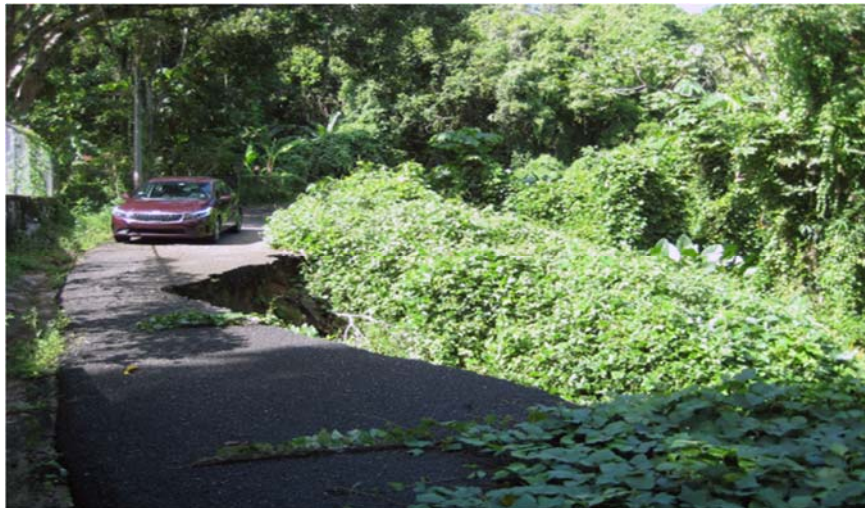
Figure 1: Collapsed Segment of Road near Maricao, Puerto Rico Source: GAO Report, GAO-19-662T, EMERGENCY MANAGEMENT: FEMA’s Disaster Recovery Efforts in Puerto Rico and the U.S. Virgin Islands
